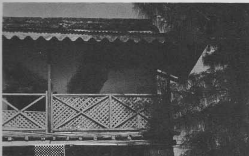
A verandah of the building pictured on this issue's cover. The National Museums plan to restore the facade this year.
